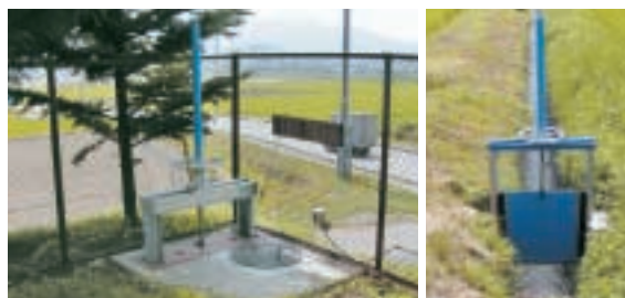
Emergency Shutoff Gate
