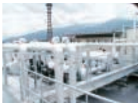
Cooling Water Pump with Higher Efficiency
