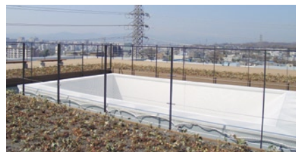
Green roof of new building of Ishikawa at the Research and Development Center in Hachioji.
