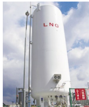
A new LNG-fueled boiler at the Tatsuno Plant
