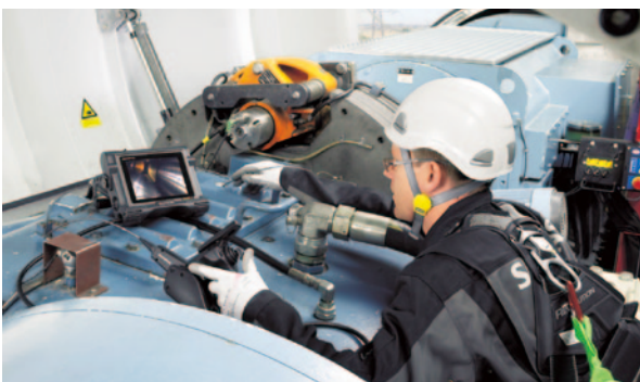
Inspecting a wind turbine generator gearbox
